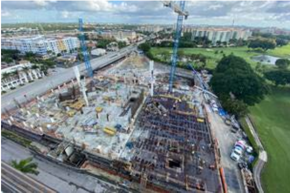
PENN-FLORIDA COS. | The construction of Penn-Florida Cos.' Residences at the Mandarin Oriental, Boca Raton.
